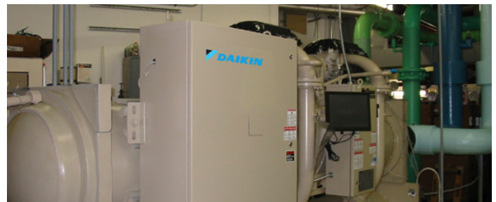
Two Daikin Magnitude magnetic bearing chillers were a part of the solution provided by Carroll Air Systems and the service department of Daikin Applied for the Philharmonic Center for the Arts.
