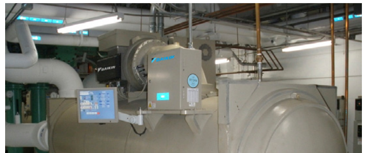
One of two 500-ton Magnitude Chillers installed at the Sarasota Bradenton International Airport
