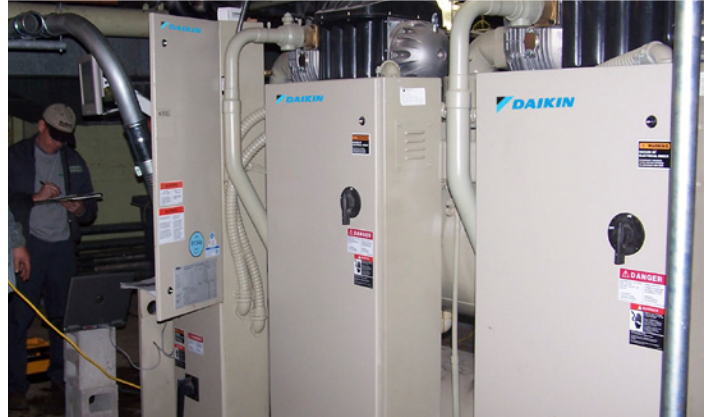
The Magnitude chiller was installed next to an older screw compressor chiller and the new chiller is dramatically quieter than the other machine.
